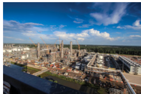
USGC Petrochemicals Project – Cedar Bayou facility in Baytown, Texas
