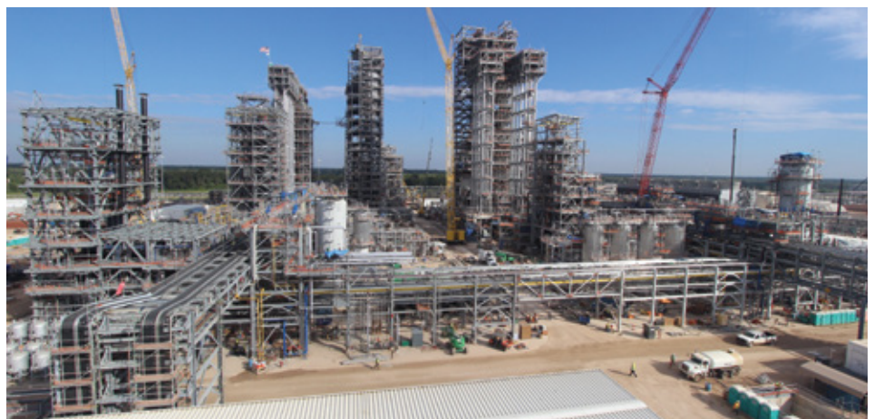
USGC Petrochemicals Project – Old Ocean facility in Sweeny, Texas
